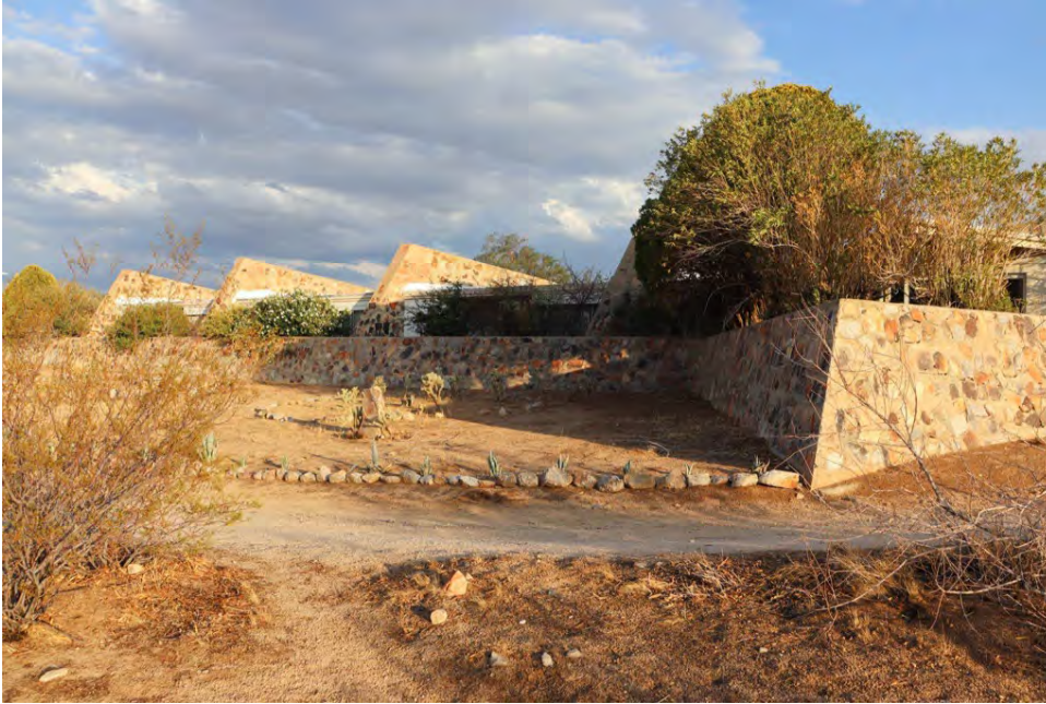
Caravansary of Joy battered wall and fin detail. View: SE. (CA_San Bernardino County_ New City of Mentalphysics Historic District_0002)
